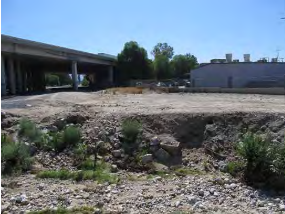
Photo 5. Looking east at the proposed Zanja Trail location below the I-10 overpass.
