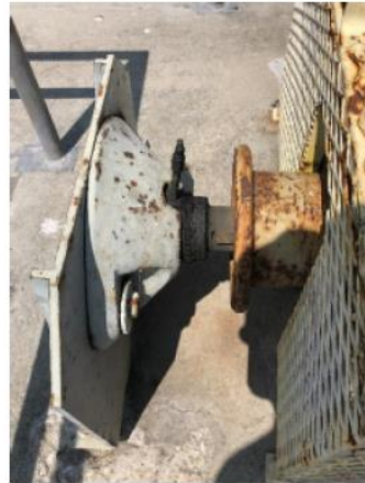
Sludge Collector Drive Primary Clarifiers 1 and 2 (1962)
