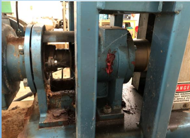
Primary Sludge Pump No. 2 (1972)
