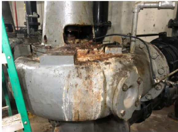
Raw Sewage Pump P-550A
