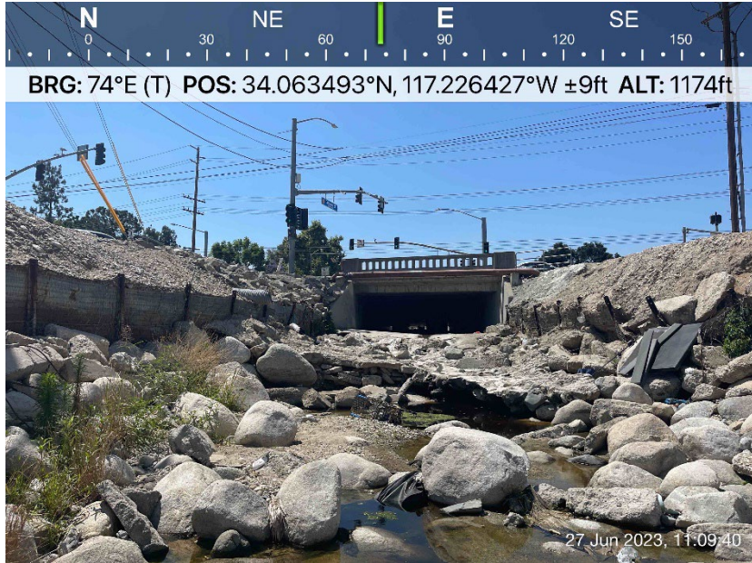
Photo Point 1. Water entering north side of intersection and end of concrete lining.
