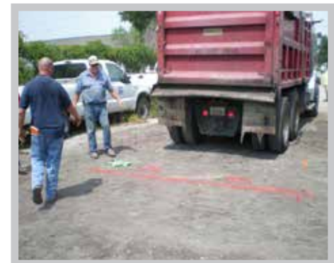
Truck (31 tons) backing over R-Tank.
