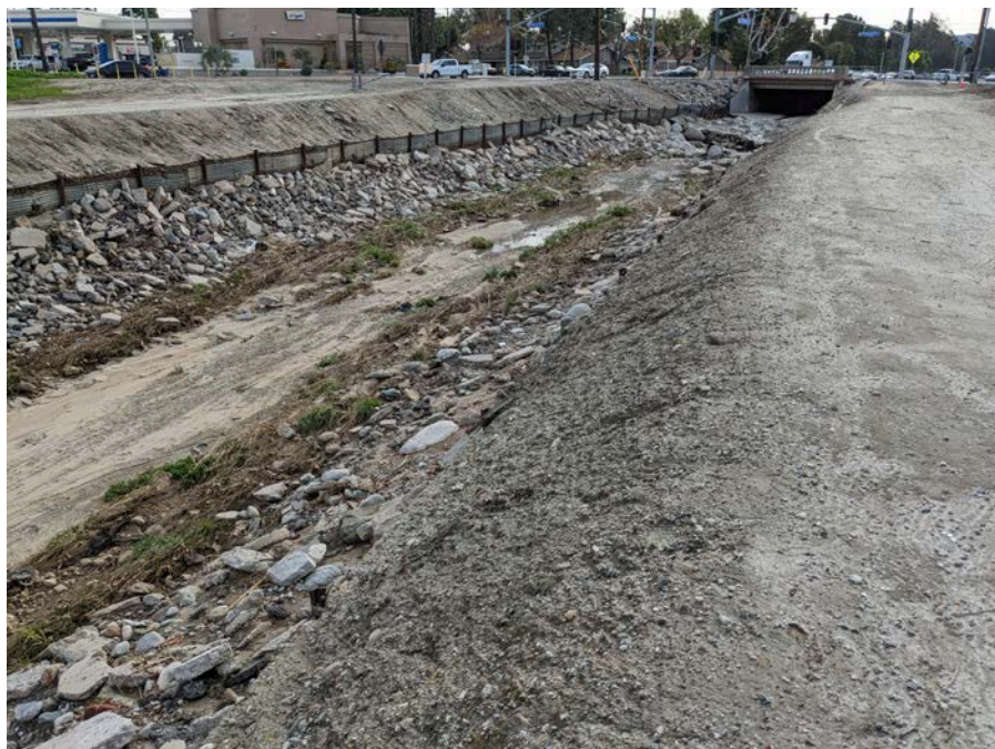
Photograph 4: View looking southeast at the Mission Creek Channel segment toward Redlands Boulevard and California Street.
