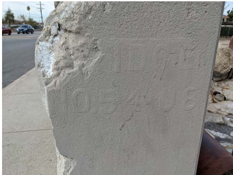
Photograph 2: Close-up of the end wall of the bridge with its numeric designation.
