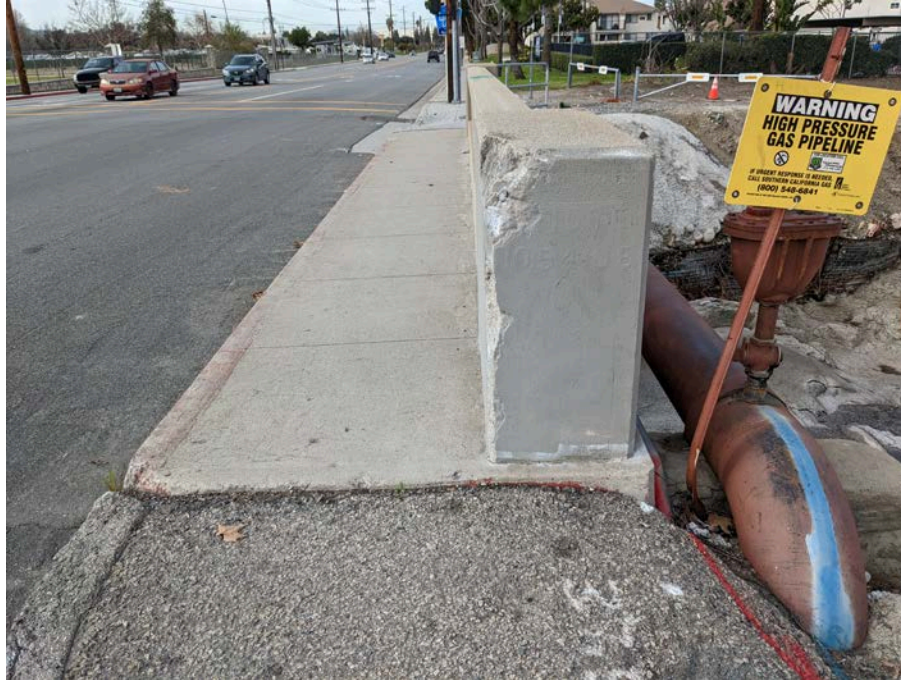
Photograph 1: View looking at the remaining part of the former reinforced concrete bridge over Mission Creek east up Redlands Boulevard on the west side of California Street.
